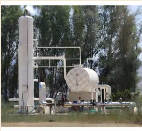
AFJET GEOTHERMAL WELLHEAD, AFYONKARAHISAR EXISTING INFRASTRUCTURE THE REPG UNIT CONNECTS TO · ORIGINAL PHOTOGRAPH
