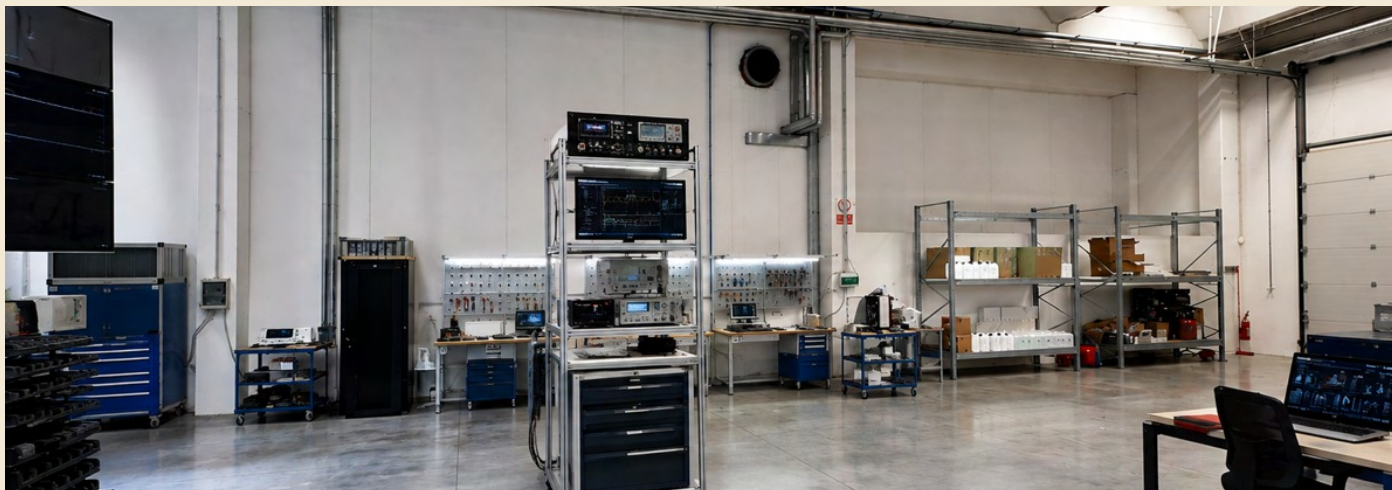
PRODUCTION HALL AND TEST FLOOR: CLEAR-SPAN AREA WITH OVERHEAD SERVICES
