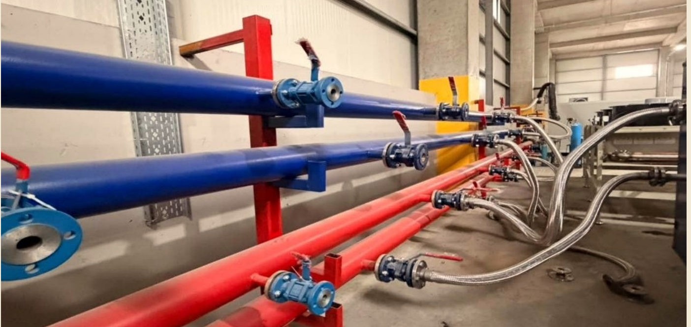
HOT AND COLD CIRCUIT PIPING AND VALVE MANIFOLD ON THE REPG TEST BENCH, BURSA
