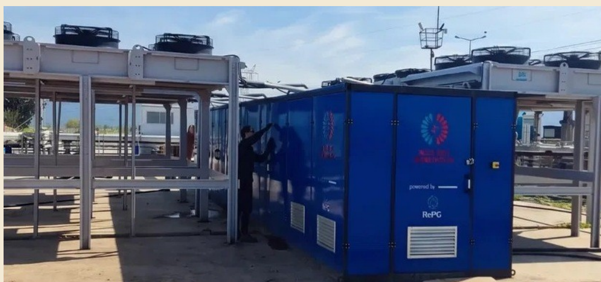
The same platform at larger scale · a 150 kWe geothermal installation delivering 100 kW net from geothermal water at 120 to 90 °C
